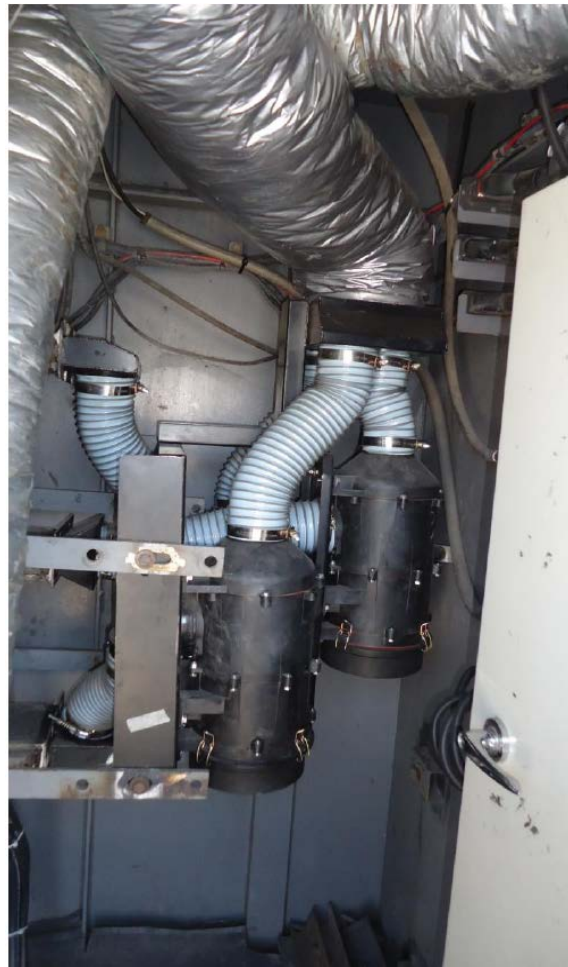
Recirculation Air Three RESPA-FFX Units
