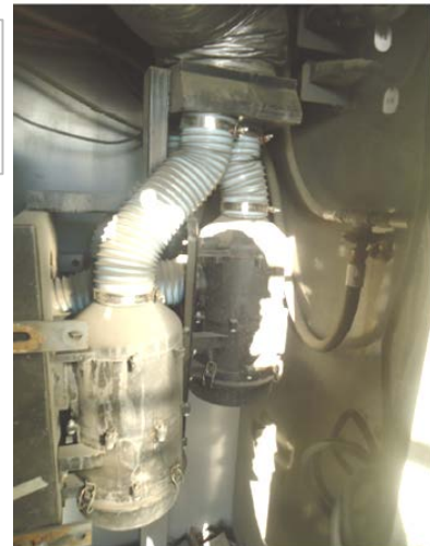
Torn door seal which caused pressure drop at 293 hours of run time. At no time during the test did the pressure ever drop below 0.35" W.G. (87 Pascal). Superior pressurization contributes to protecting the cab and operator from dust infiltration.
