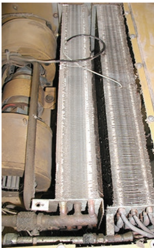
A. Before the installation of a cab air quality system, the fins in the HVAC evaporator coils are clogged with debris and a layer of dust covers the compartment.
