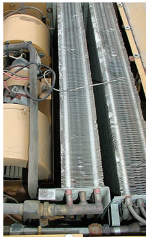
B. One year after the installation of a cab air quality system, the fins in the HVAC evaporator coils are clean and the compartment is not dusty.
